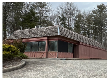
Mansard Roof (inconsistent)
