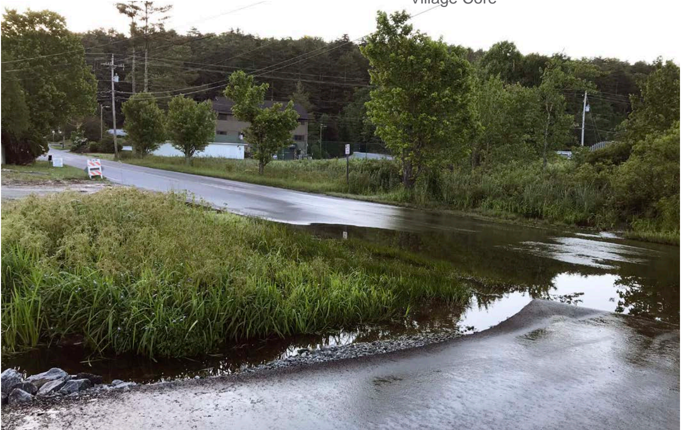
Poor drainage along Frank Allen Road results in a perpetual flow of ground and stormwater. This issue presents a safety hazard and is a significant barrier to walking
