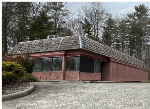
Mansard Roof (inconsistent)
